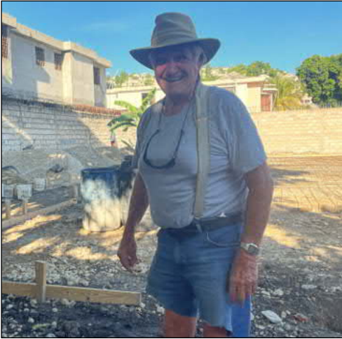
Tech Serve Volunteer Larry Zaugg building the slab for the trade school building in Haiti.
